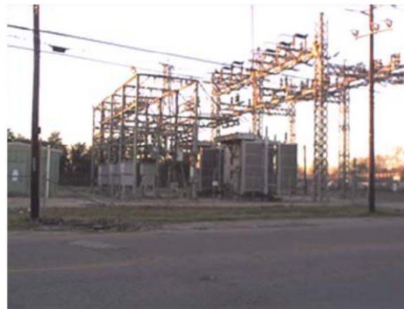
Transformers and Substations
